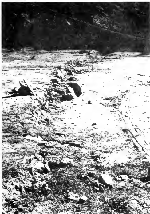
Photo 15. Veterans fault scarp where it was best developed east of the corner of Tucker Avenue and Rejah Street. Scarp is 15 cm (6 inches) high across a graded bedrock surface. Pencil leaning on scarp for scale.
